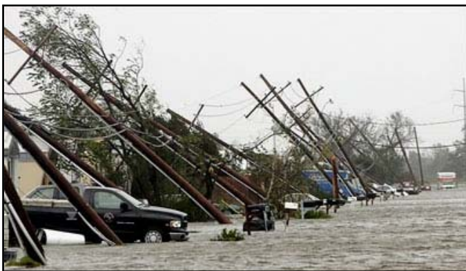
Power lines damaged by hurricane Katrina
